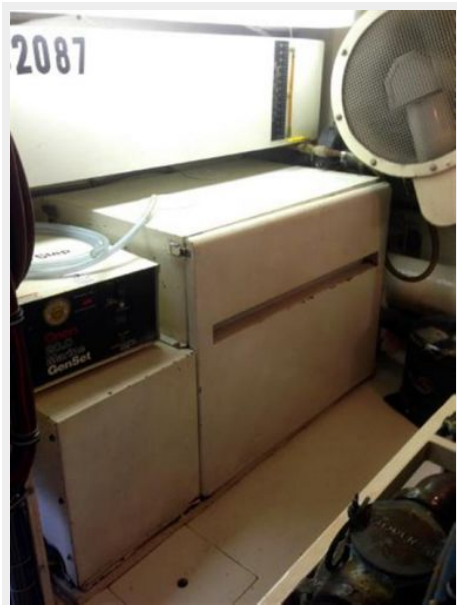
Engine Room - Genset
