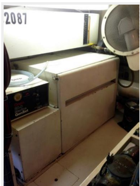
Engine Room - Genset
