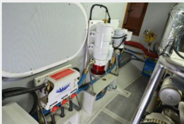
Fuel tank starboard with ESI Fuel polishing system
