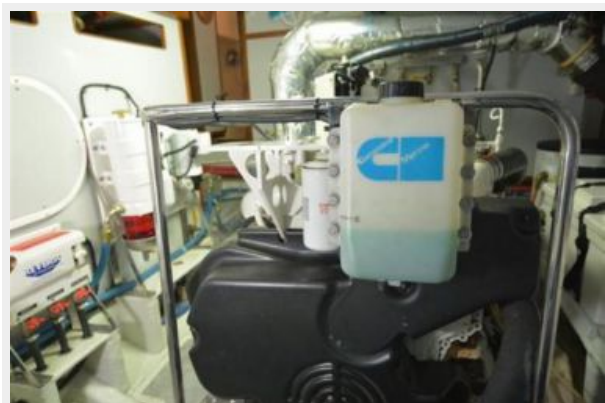
Engine room- Looking aft
