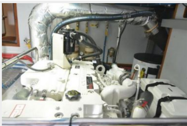
Engine room- Looking aft
