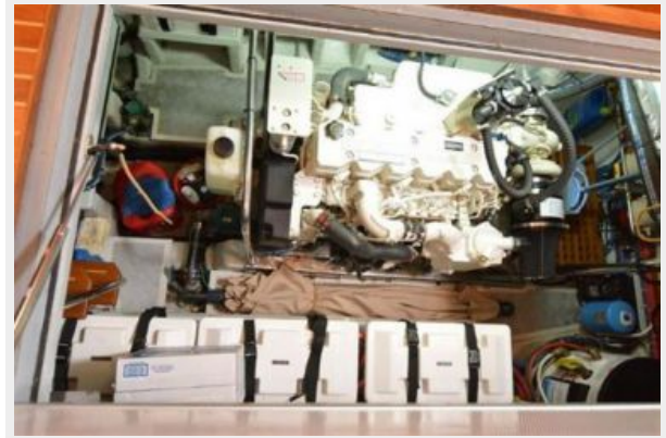
Engine room looking down from open hatch
