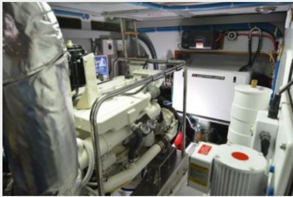
Engine room- Looking forward
