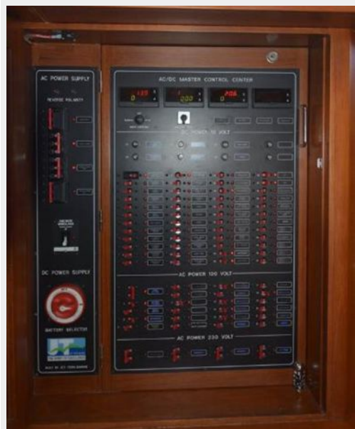
Selene electrical distribution panel
