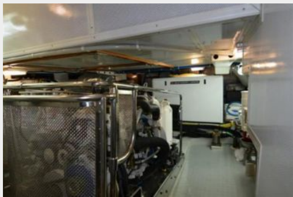
Engine room- Looking aft
