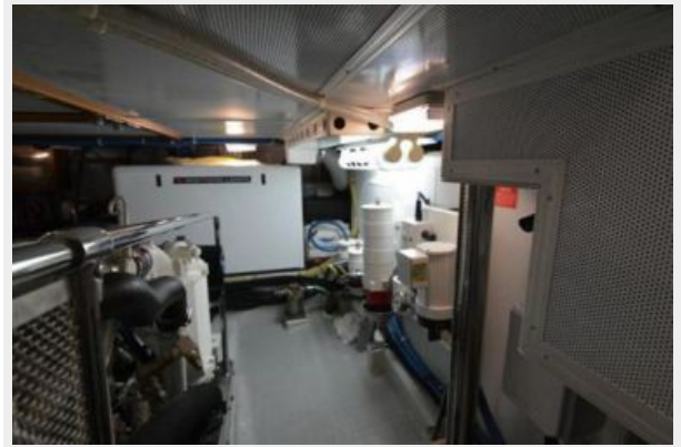
Engine room- Looking aft
