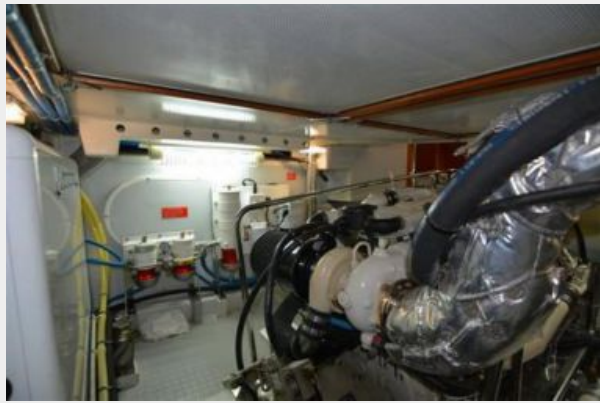
Engine room- looking to port
