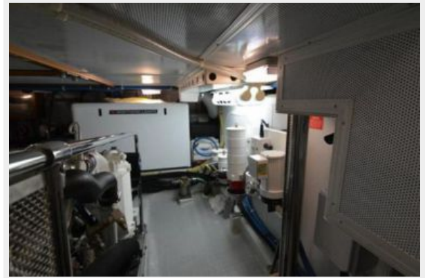
Engine room- Looking aft
