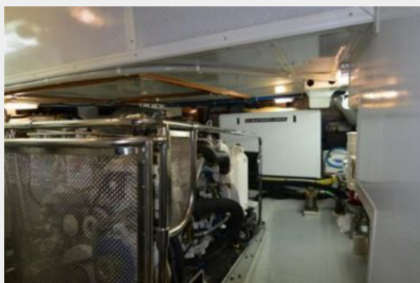
Engine room- Looking aft
