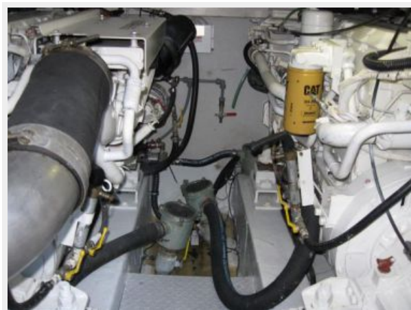
Clean Engine Room
