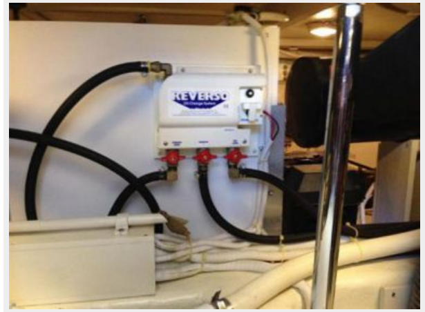
Oil exchange system for mains and genset
