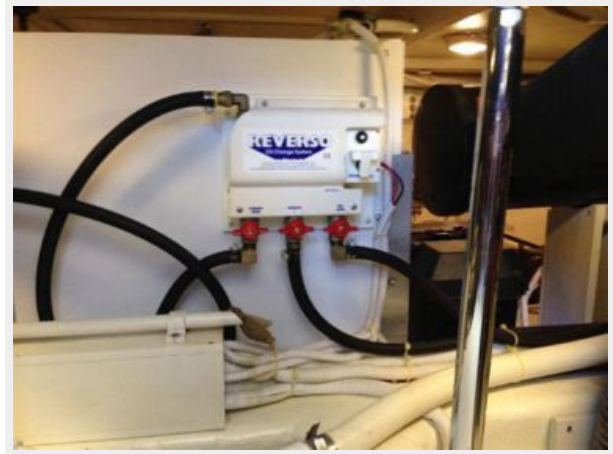
Oil exchange system for mains and genset
