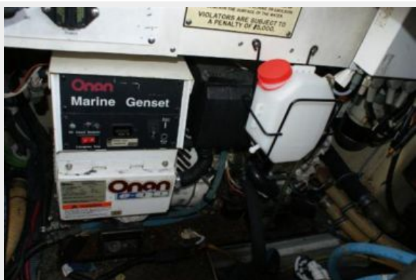
Onan 7.5KW genset
