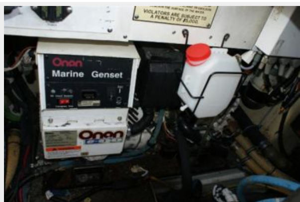
Onan 7.5KW genset
