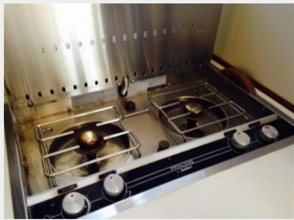
Gas burners under
