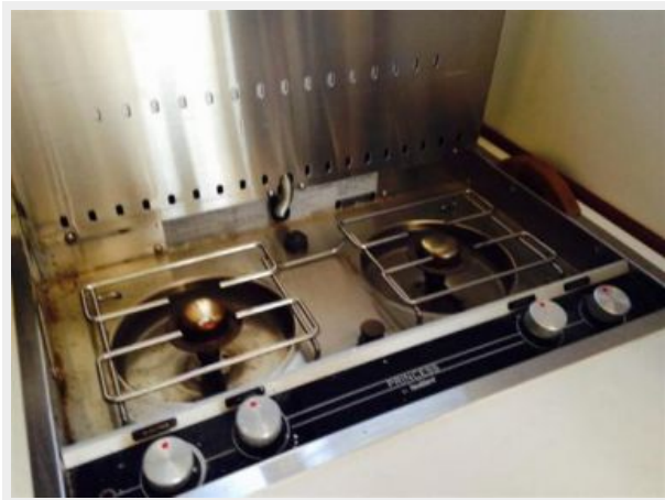
Gas burners under
