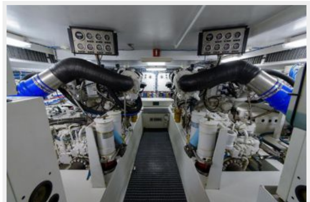
Engine Room Looking Forward
