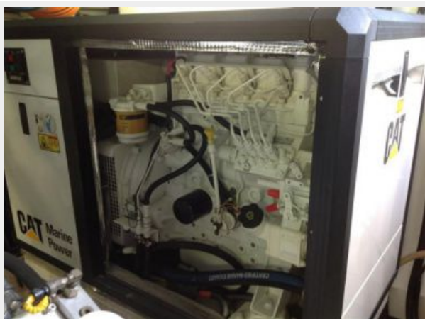
24.3 KW CAT Generator
