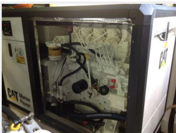
24.3 KW CAT Generator
