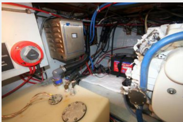
Generator / Battery Charger
