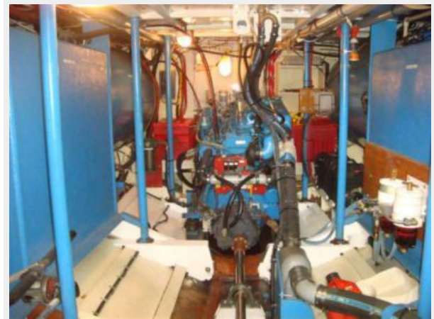
46' Roberts engine room forward
