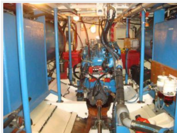
46' Roberts engine room forward
