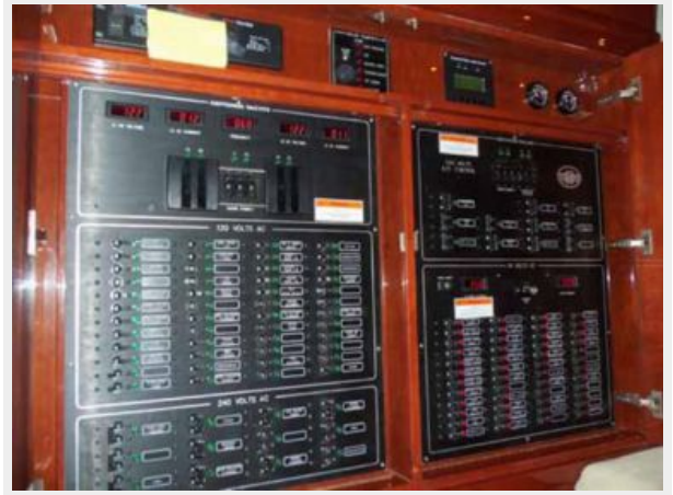
Electrical Locker in Companionway
