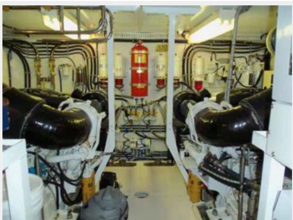
Engine Room Looking Forward
