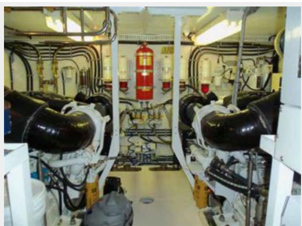
Engine Room Looking Forward
