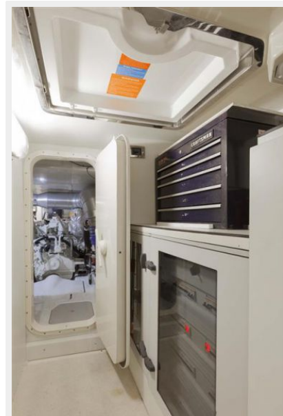
Engine Room Entrance
