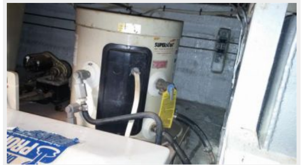
Hot Water Tank
