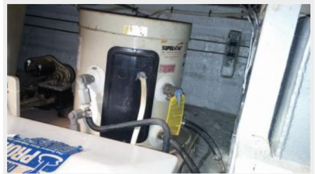
Hot Water Tank
