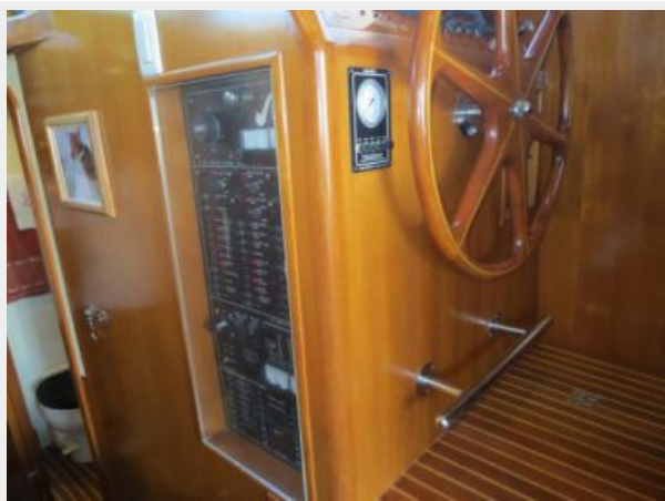
Lower Helm/Electrical Panel
