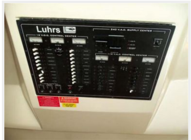
Overhead Electrical Panel
