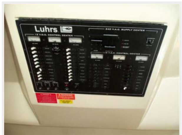
Overhead Electrical Panel
