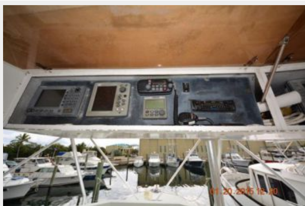
Flybridge electronics box
