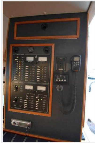
Electric Panel and Cabin VHF
