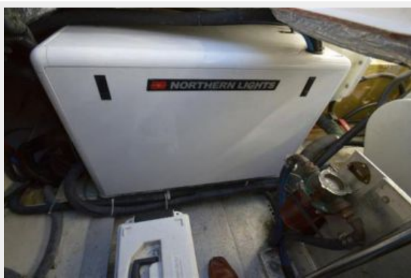
Generator in Sound Shield
