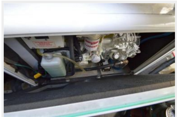
Generator Inside Sound Shield
