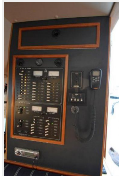
Electric Panel and Cabin VHF
