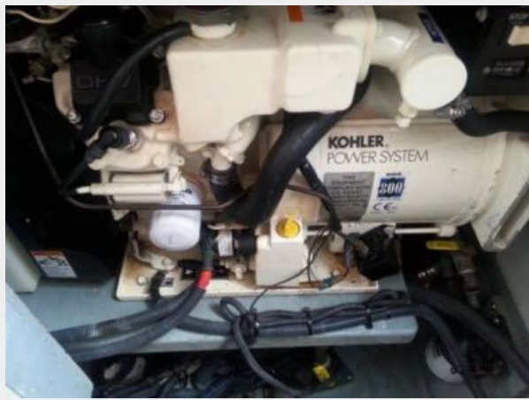
5KW Kohler Genset
