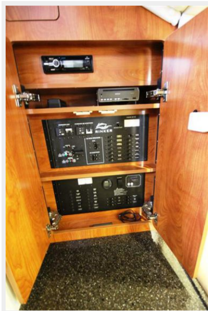
Main Distribution Panel
