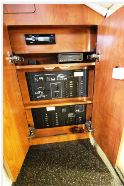
Main Distribution Panel
