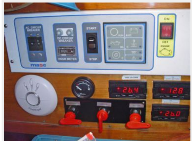
Generator Electrical Display
