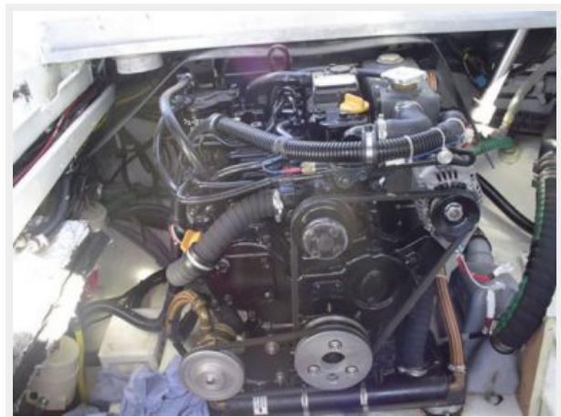
Mase/Yanmar IS9 230AC 50 htz 8.5KW Generator
