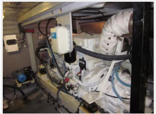
Engine Room Stb
