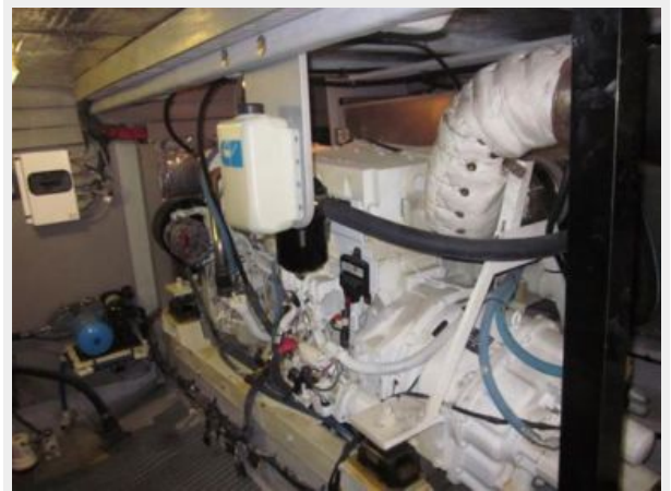
Engine Room Stb
