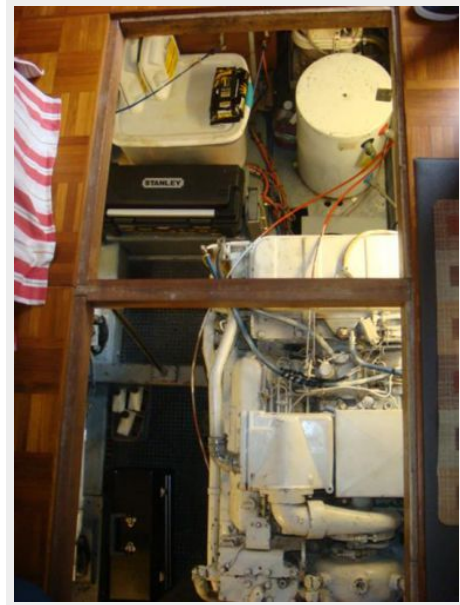
52' Jefferson engine room
