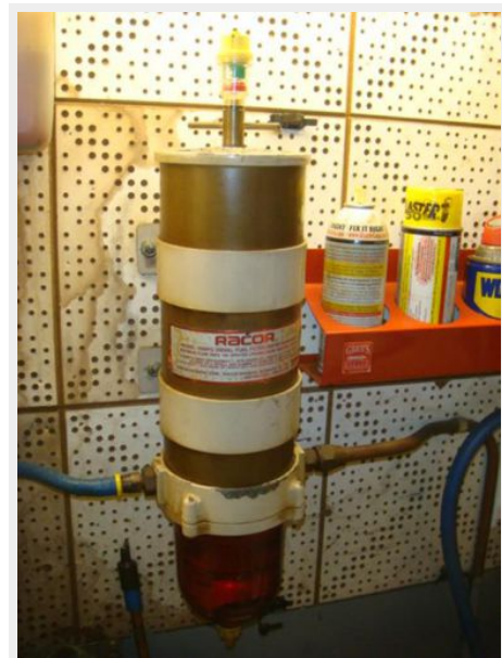
52' Jefferson starboard main engine Racor fuel filter
