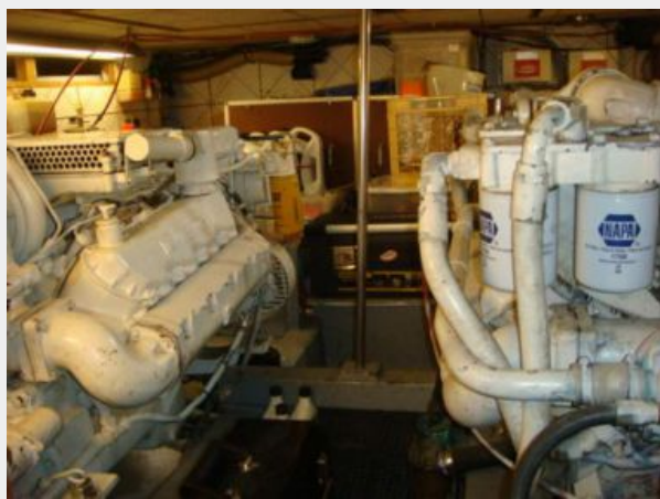
52' Jefferson engine room forward
