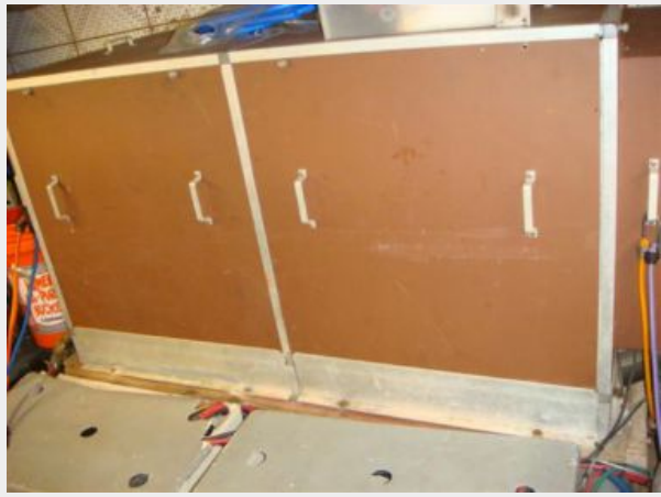
52' Jefferson generator sound box
