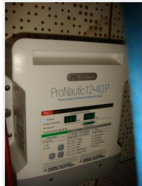
52' Jefferson battery charger
