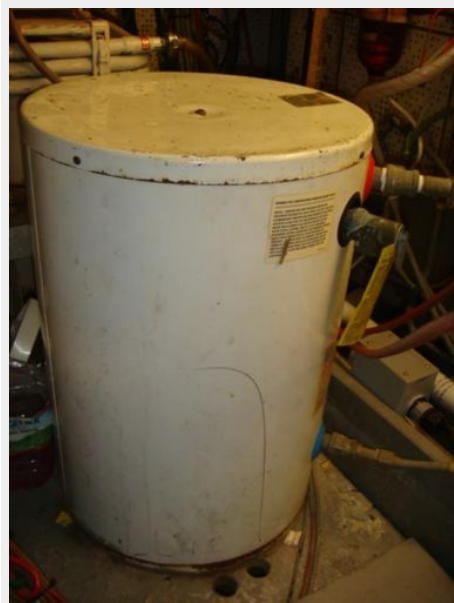
52' Jefferson water heater
