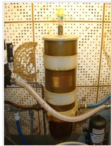
52' Jefferson Port main engine Racor fuel filter
