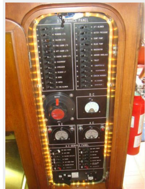
52' Jefferson electrical panel
