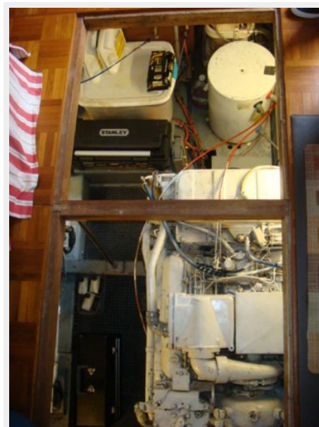
52' Jefferson engine room
