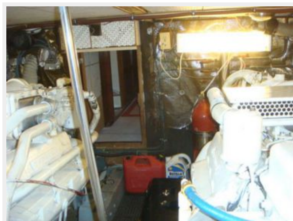
52' Jefferson engine room aft
