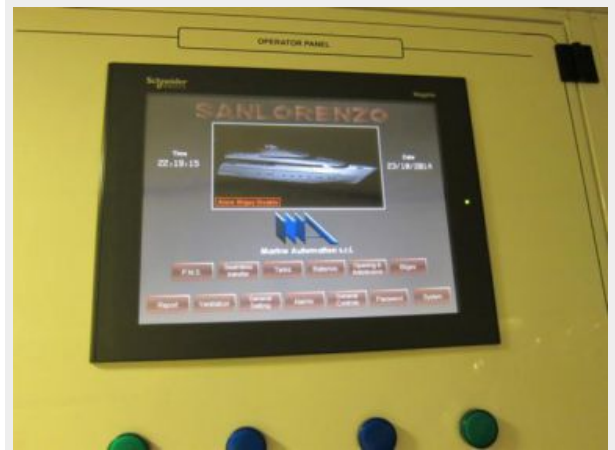
San Lorenzo Control Panel
