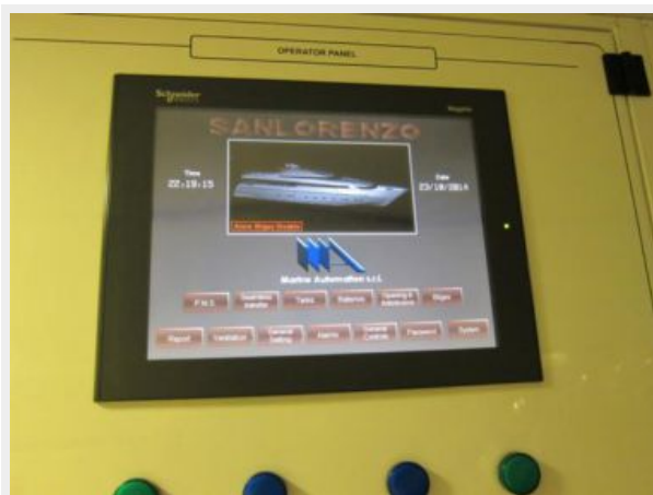
San Lorenzo Control Panel
