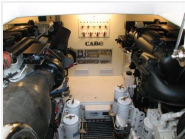
Engine & Mechanical Equipment 1 - Engine Room
