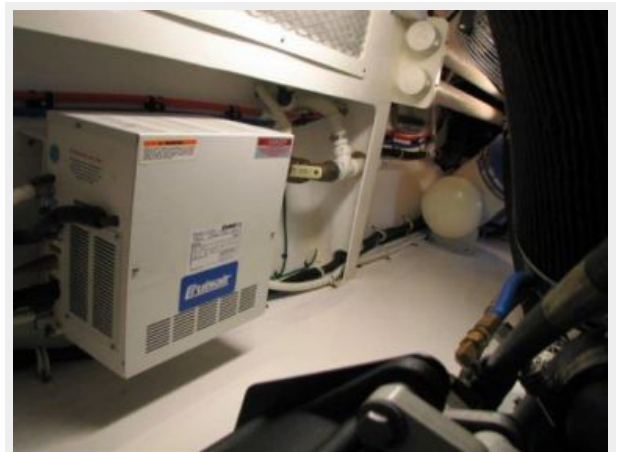
Engine & Mechanical Equipment 6 - Engine Room
