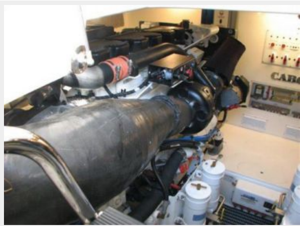
Engine & Mechanical Equipment 3 - Port Engine
