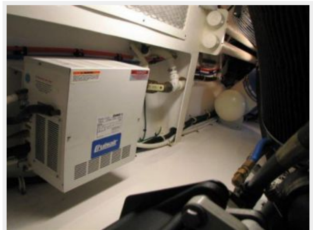
Engine & Mechanical Equipment 6 - Engine Room
