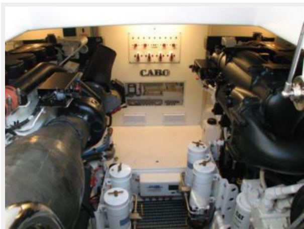
Engine & Mechanical Equipment 1 - Engine Room
