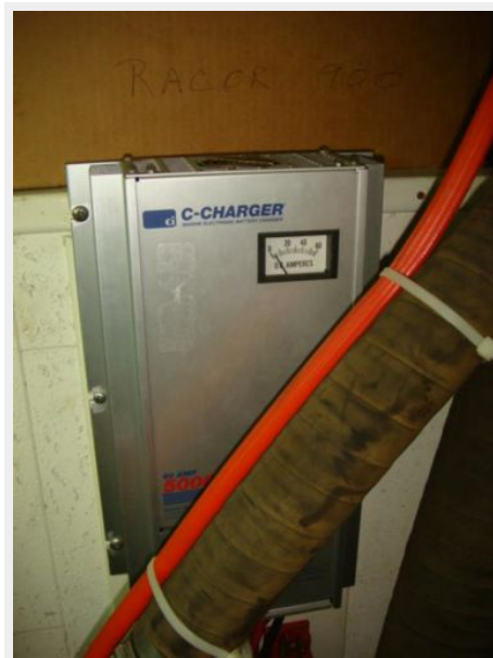
44' DeFever Battery Charger 2
