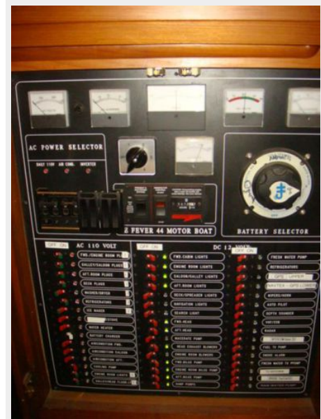
44' DeFever Electrical Panel
