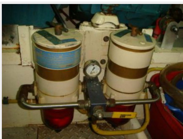
44' DeFever Starboard Racor Fuel Filters
