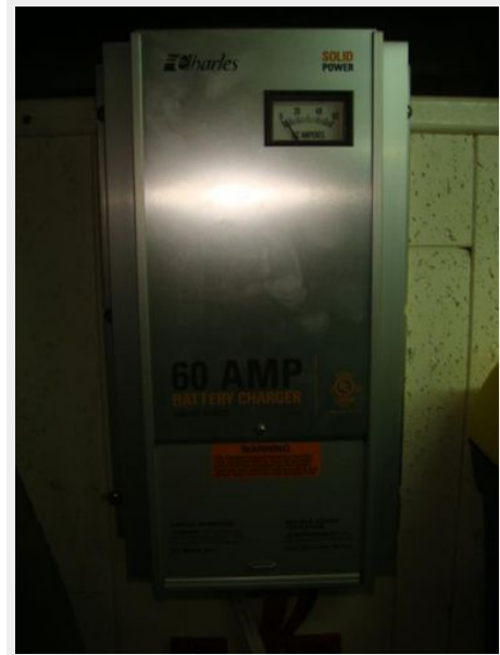
44' DeFever Battery Charger 1
