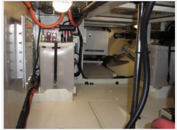
Engine Room Looking Aft
