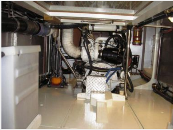
Engine Room Looking Forward
