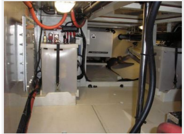
Engine Room Looking Aft
