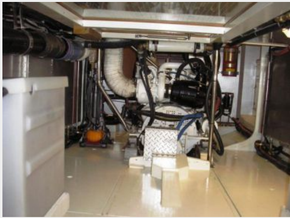
Engine Room Looking Forward
