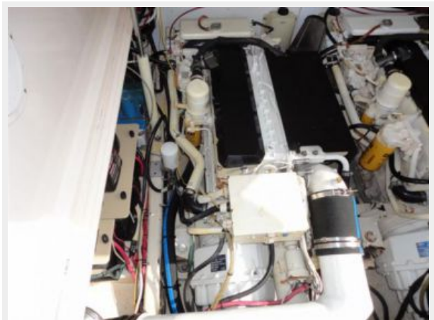
Outboard Side Port Engine
