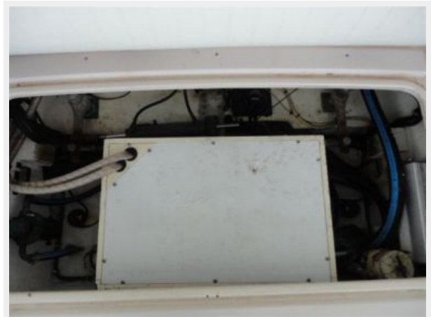
Generator Sound Shield
