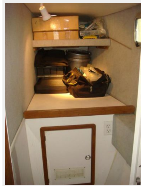
36' Endeavor Starboard Forward Generator Room
