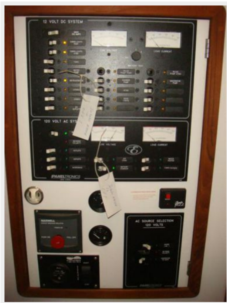
36' Endeavor Electrical Panel
